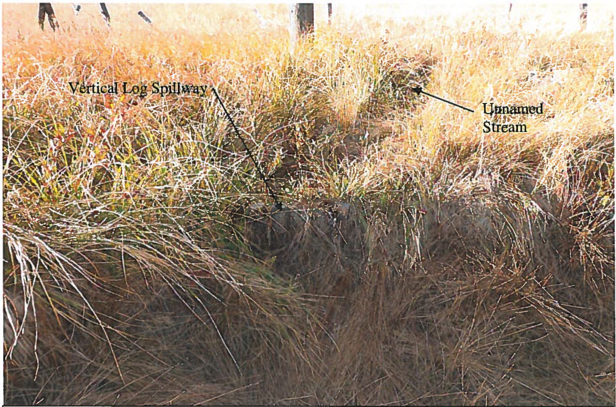
View southerly of 'log' spillway for storage pond. Water discharges southerly through the vertical log sections to the unnamed stream.
