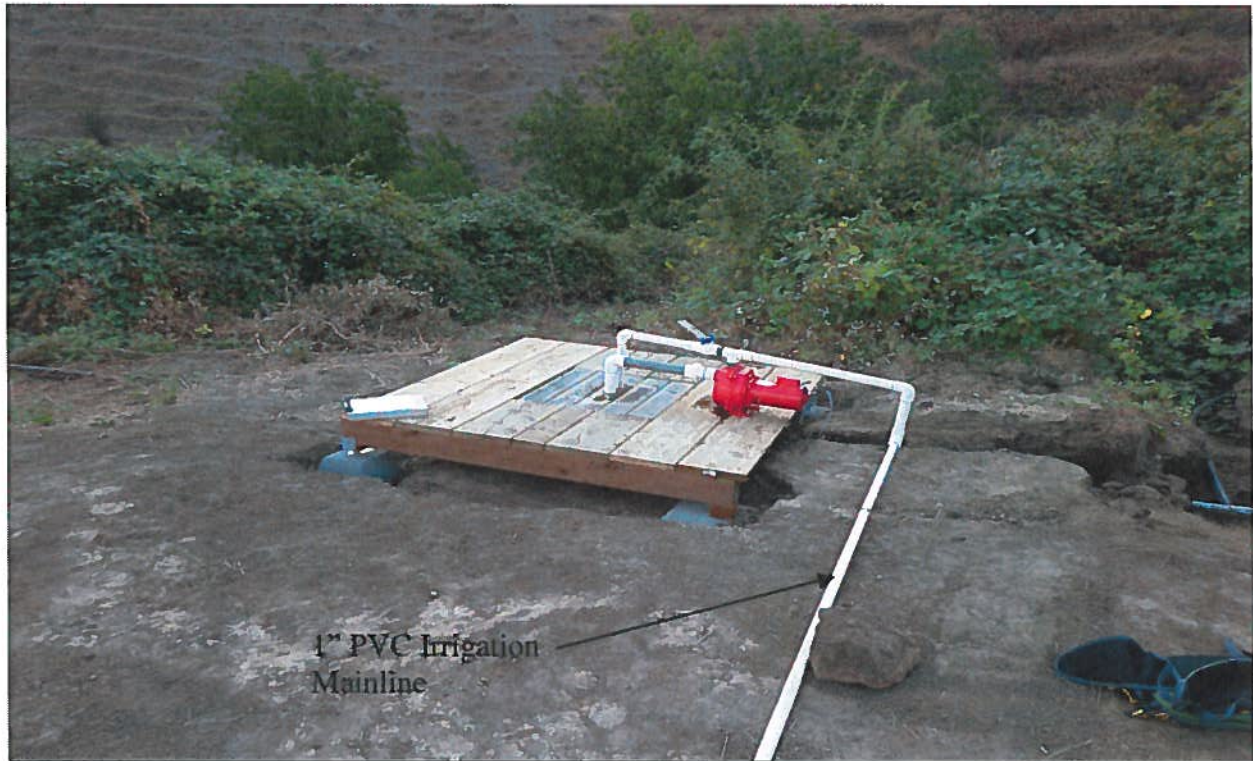
View easterly of the pumping platform over the buried 1,400 gallon irrigation water storage tank filled by the 1 1/2" polypipe in Elfers Creek. A 1 hp pump diverts water through the 1" PVC mainline to the garden area irrigation sprinkler system.
