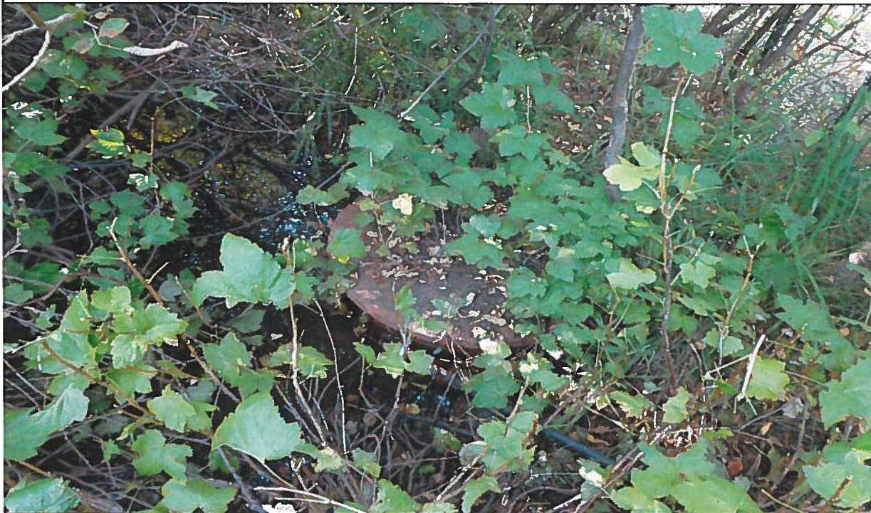
Point of Diversion: View of 3-foot diameter spring box. The spring box is sealed with a lockable steel lid.
