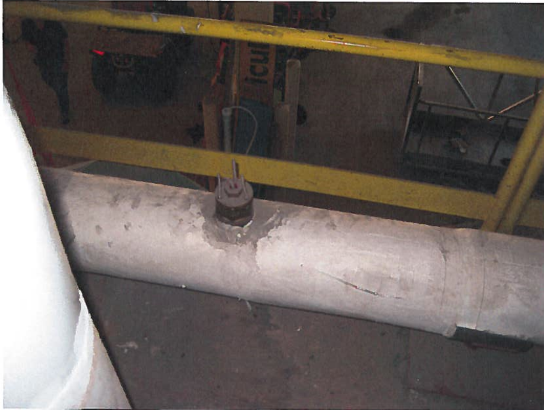
In line impeller Measuring device (replaced 2012 after my visit)
