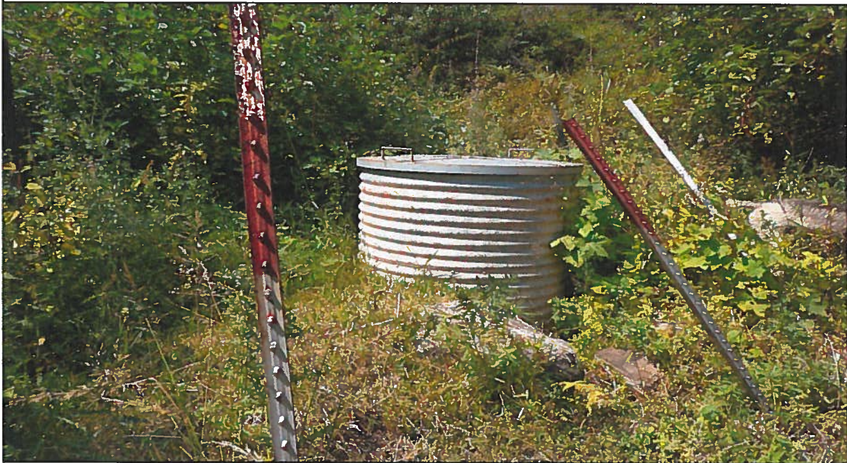
Point of Diversion: View southwesterly of 4' diameter CMP spring box. Approximately 480 lineal feet of 1" PVC pipe conveys water to an excavated channel to a stock water storage pond.
