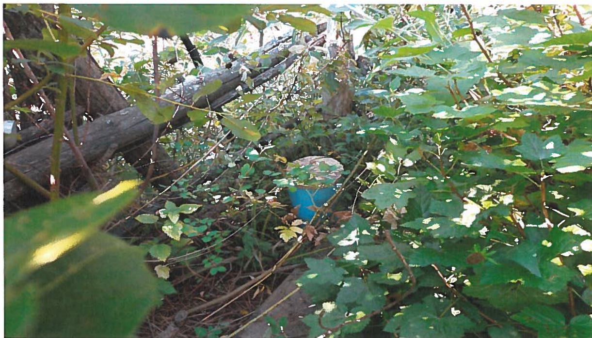
Point of Diversion (Neighbor's Cabin): View of valve box located approximately 6' south of the spring box. Although unable to confirm with the right holder, and since the spring is shared with the neighbor, it is assumed that the valve box contains the flow control valve to the neighbor's cabin.
