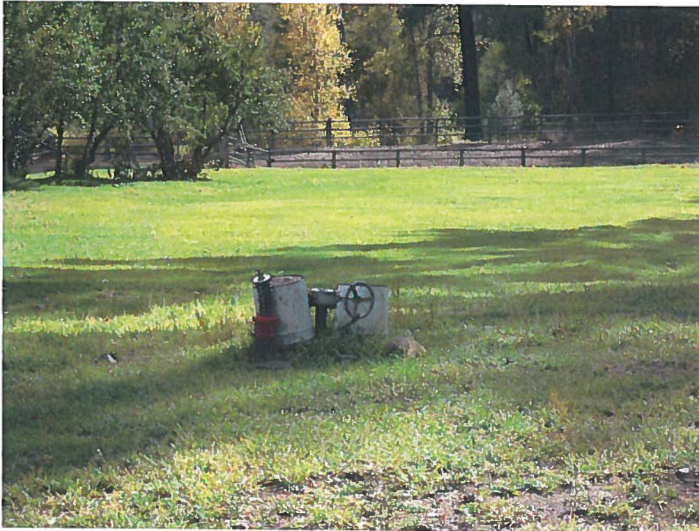
The water pipe and the electrical system share the same trench parallel to Indian Creek on the west side. This is at the upper end, downhill from the building on the previous page.
