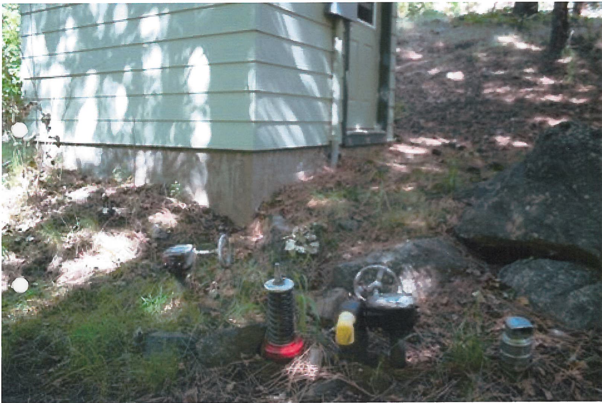
Turbine house valves. JFG
