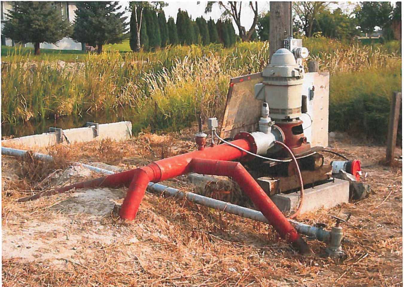
Canal Water Pump
