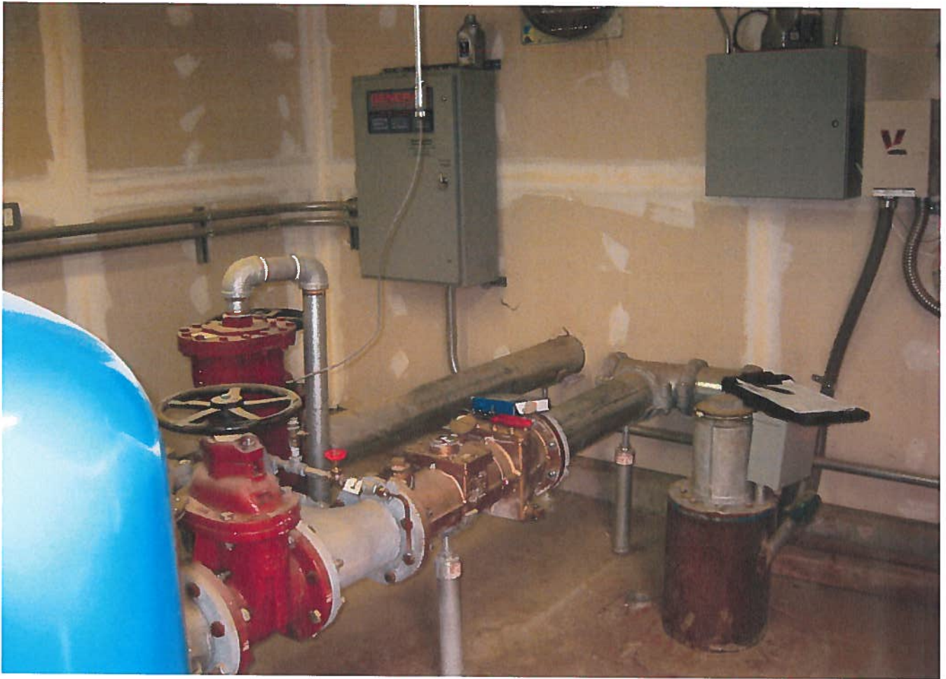
Plumbing inside North wellhouse and north wellhead.
