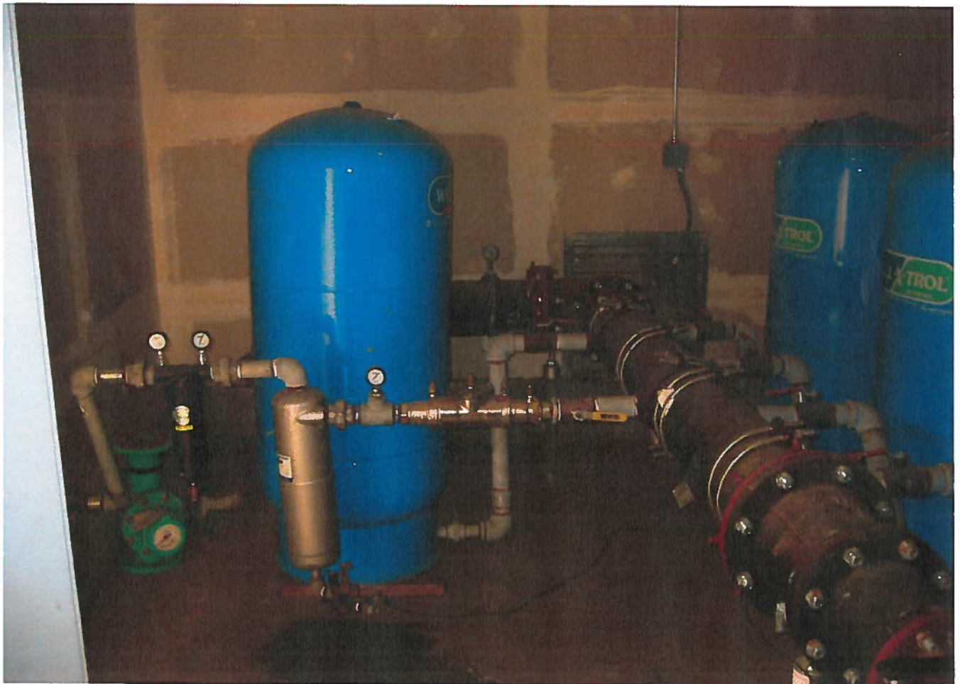
Inside south well house
