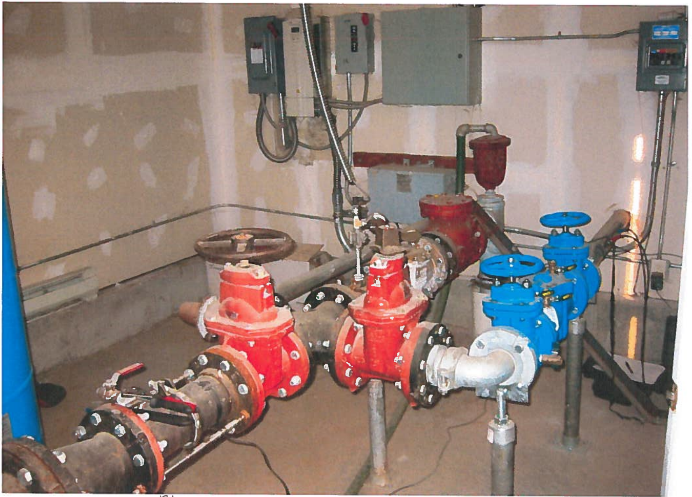
Plumbing inside south wellhouse
