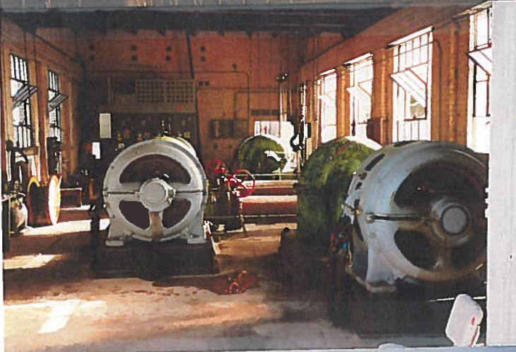
↪ Turbines inside pump station
