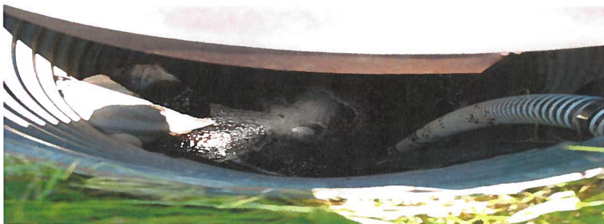
Return flow tank at Pond 2
