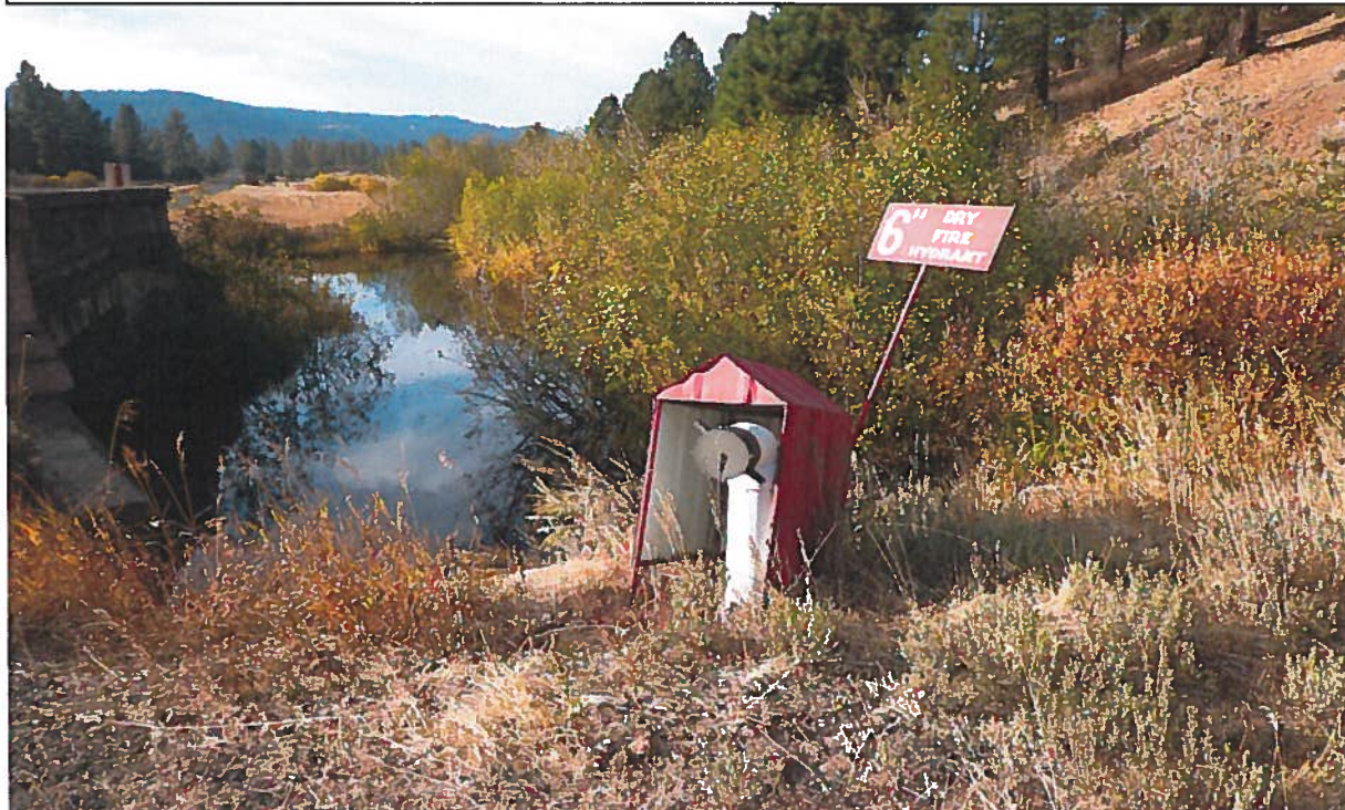
Point of Diversion: View northwesterly of 6" dry fire hydrant and Mud Creek. A 6" screened PVC pipe suction line extends along the bottom of Mud Creek.
