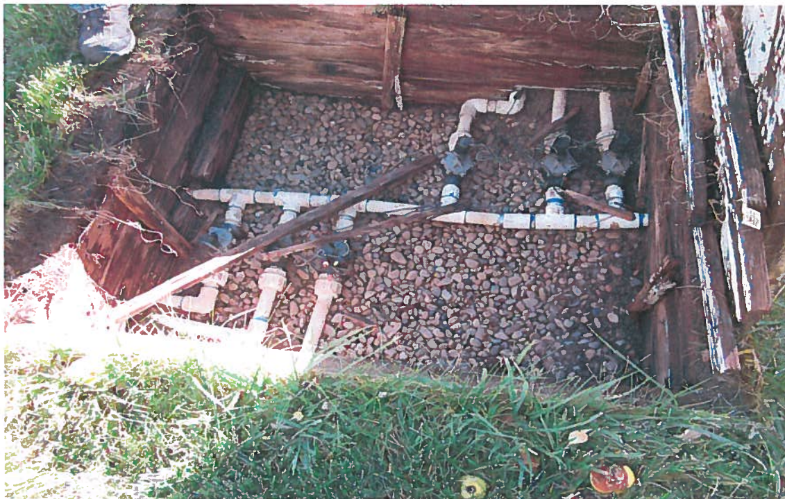
Piping from well to house for internal domestic and sprinkler system.
