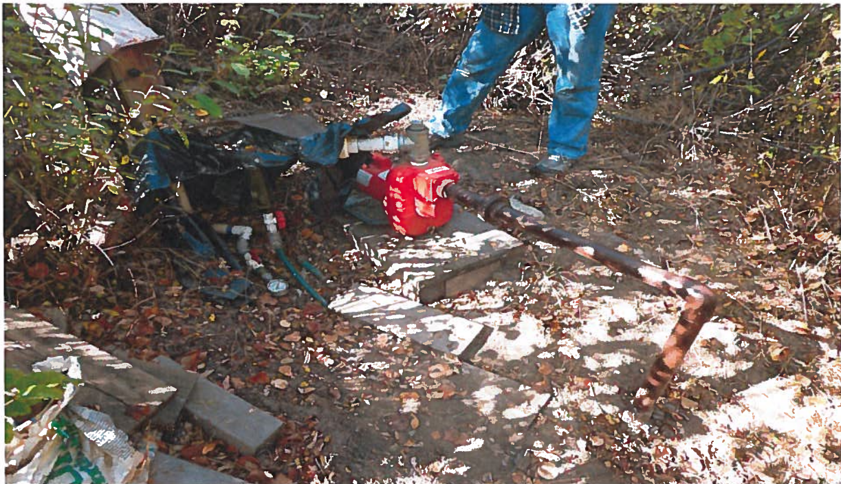
View southwesterly of a 1-hp Red Lion pump and the 1 1/2" steel pipe suction line on top of the bank of Warm Springs Creek.
