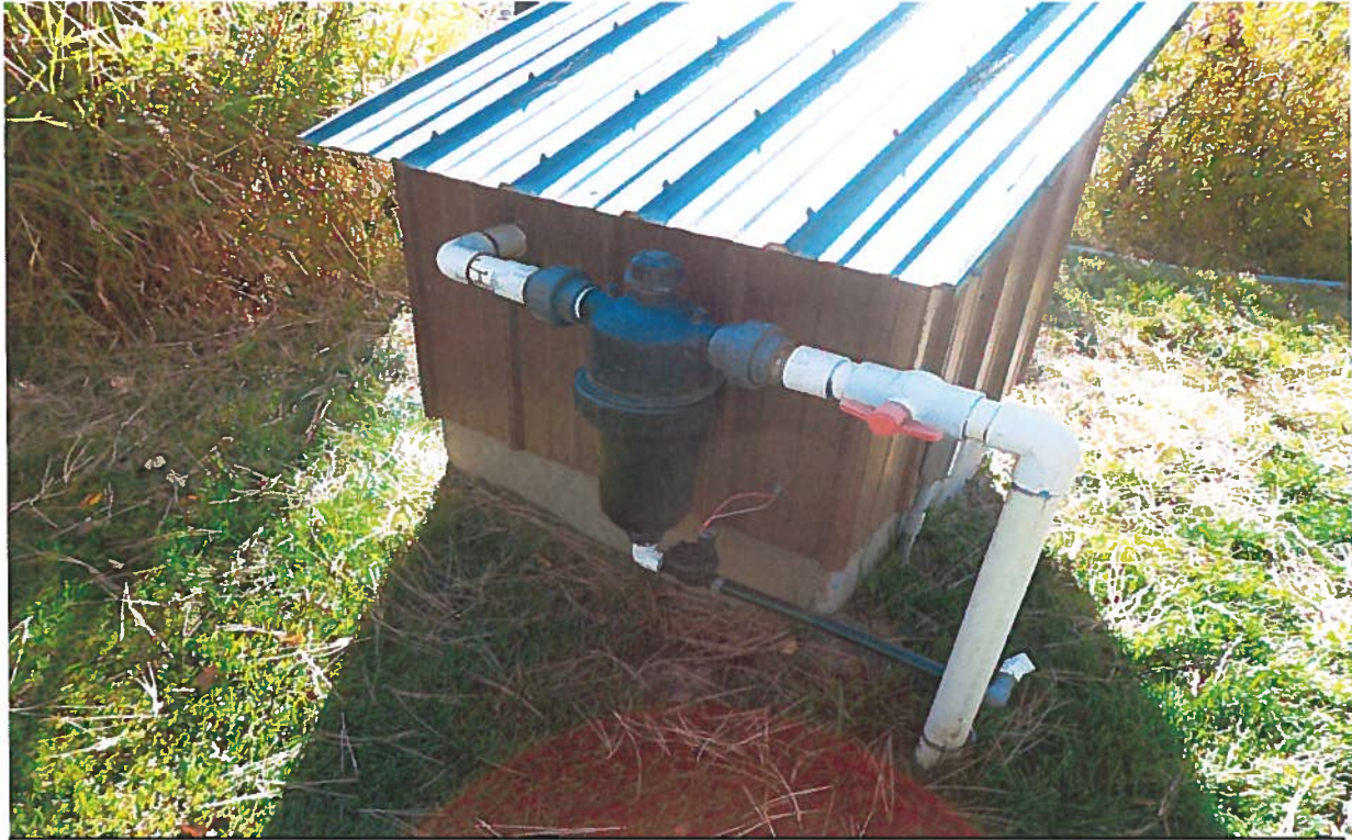
View behind the pump enclosure structure of the irrigation main line filter and a solenoid valve controlled drain line for flushing the filter.
