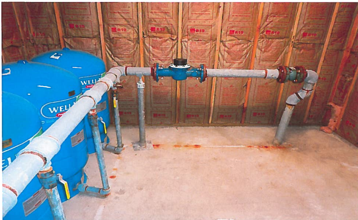
View inside of well house of the 3" galvanized supply line from the well, an AMCO Volumetric Flow Meter, and pressure tanks.
