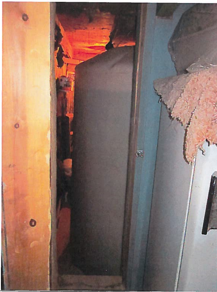
The 3,000 gallon tank for domestic water storage is in a room off the attached garage.
