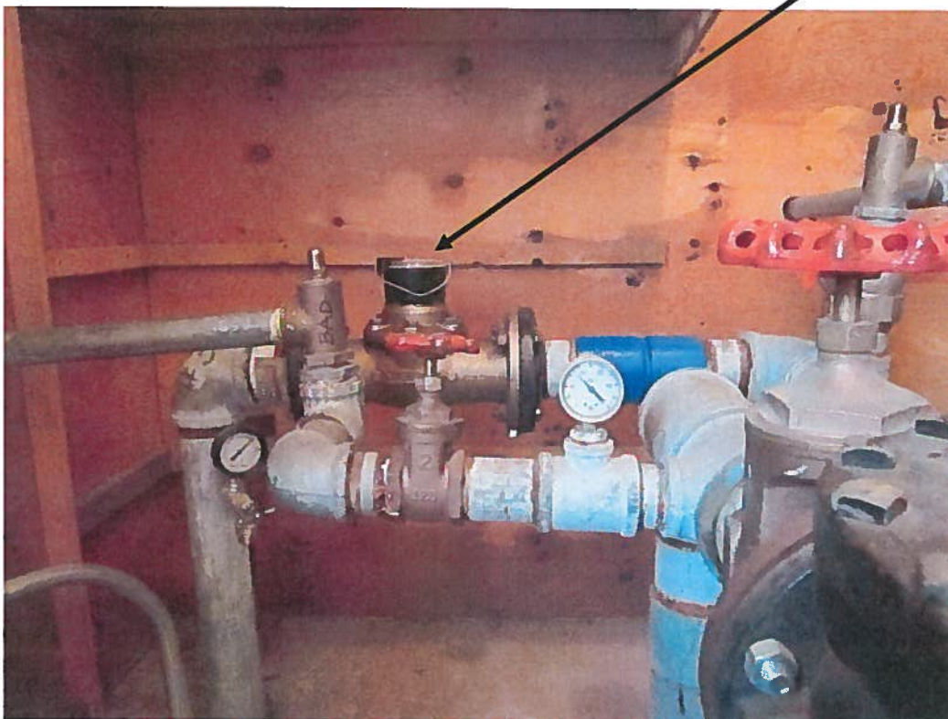
Piping for well 3
