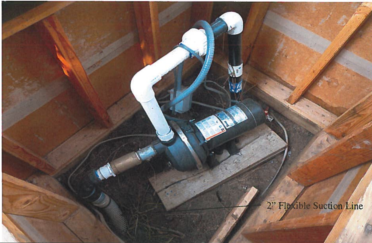
View inside of pump enclosure of the 2" flexible suction line from the unnamed stream and the 1 1/2 - hp pump and 1 1/2" PVC discharge line.
