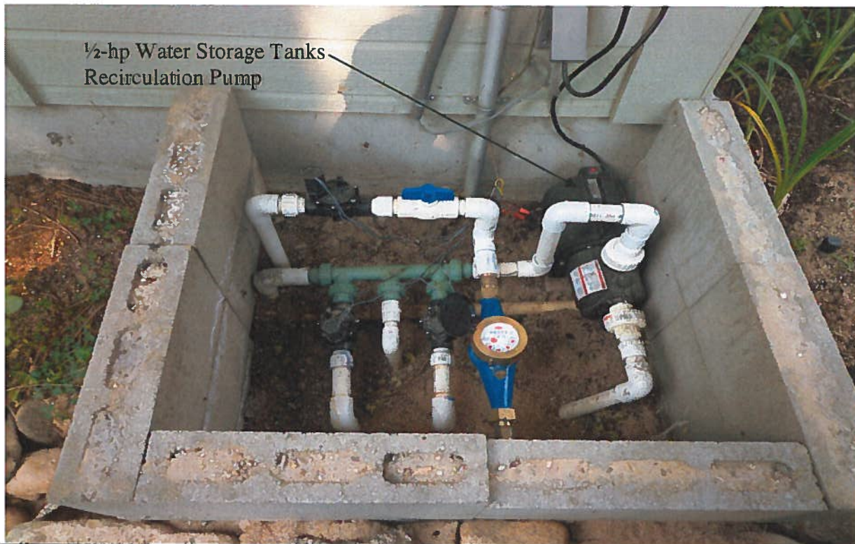
View of 1" PVC irrigation distribution main lines in a concrete block distribution vault next to the home. The 1/2-hp pump in the vault pumps water to two 2,000 gallon fiberglass water storage tanks (Water Right Permit No. 65-22942).
