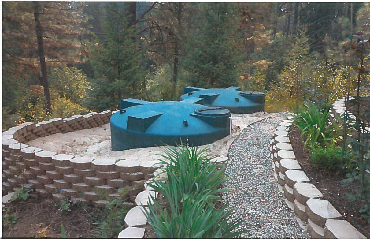
View southerly of two (2) 2,000 gallon fiberglass irrigation water storage tanks.
