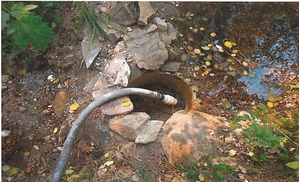
Point of Diversion: View into 24" diameter PVC cistern or sump of the 2" screened flexible suction pipe.
