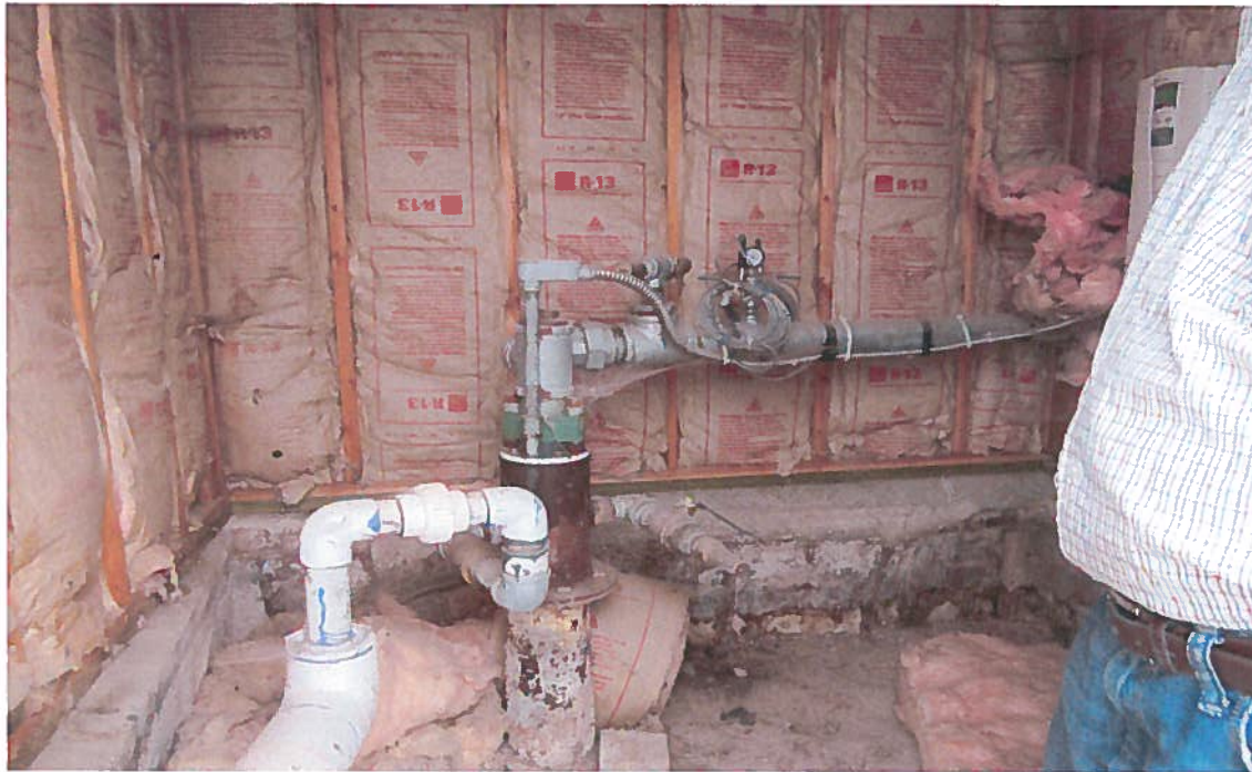
6" artesian well inside pump house.
