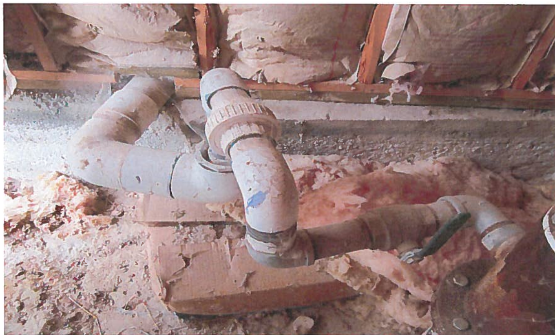
Steel and PVC piping from well.
