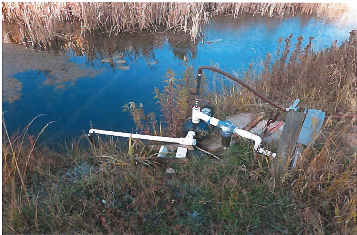
View westerly of 1 ½" PVC suction line and a 2-hp pump diverting water from a pond. Water is discharged through a 1 ½" PVC supply line to the pressurized irrigation system for irrigation of lawn, landscaping, and garden areas.
