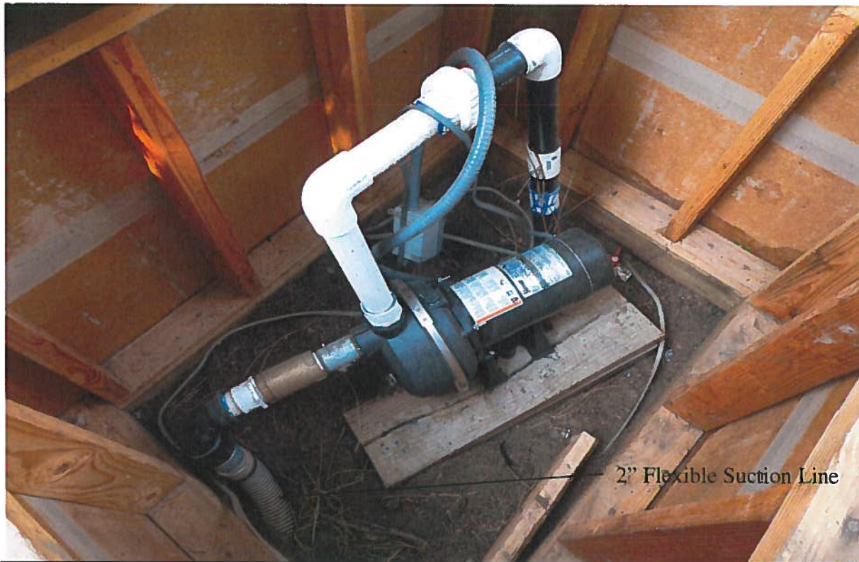
View inside of pump enclosure of the 2" flexible suction line from the unnamed stream and the 1 1/2 - hp pump and 1 1/2" PVC discharge line.
