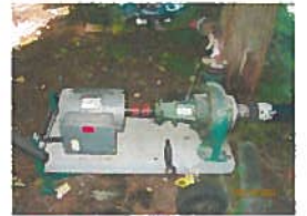
irrigation pump 5 hp.JPG
