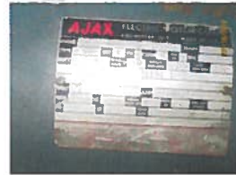
IRRIGATION PUMP TAG.JPG
