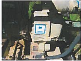
PUMP FROM CREEK
