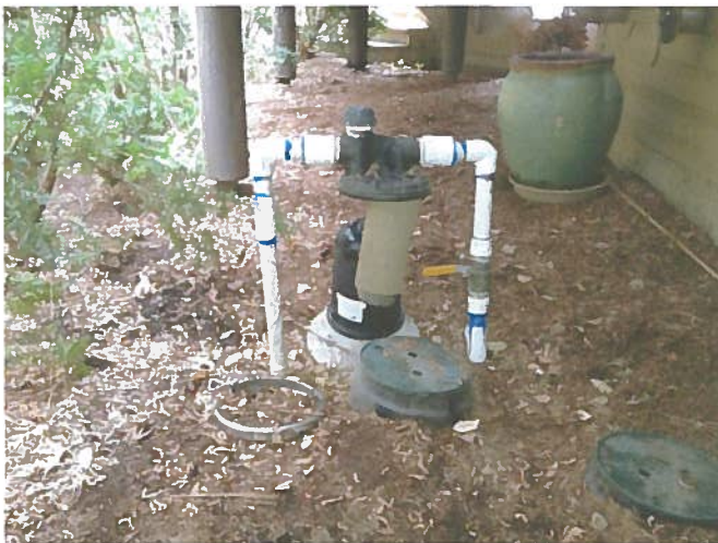
Pump control box under deck
