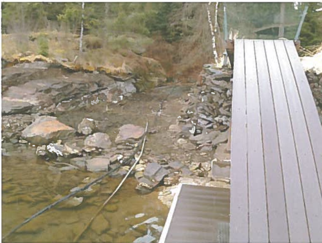
1 1/4" discharge line and 1" power feed
