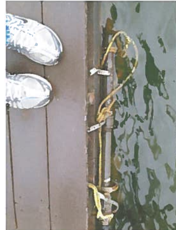
1 1/4" Discharge line and yellow retrieval line
