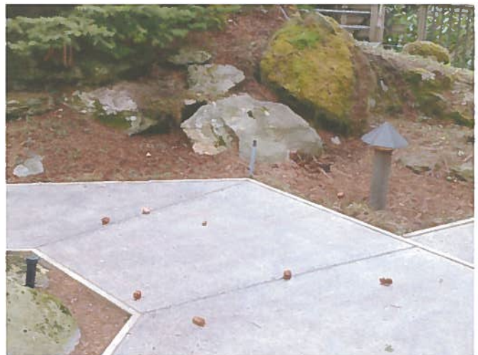
Sprinkler heads typical of u/a irrigation system
