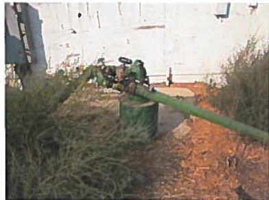
The photo above is the Vet 4 well
