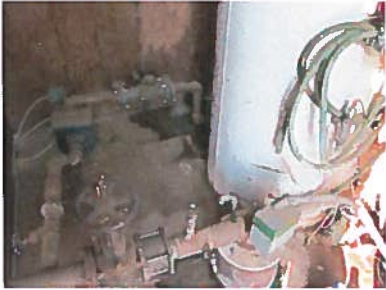
The photo above is the Highway well
