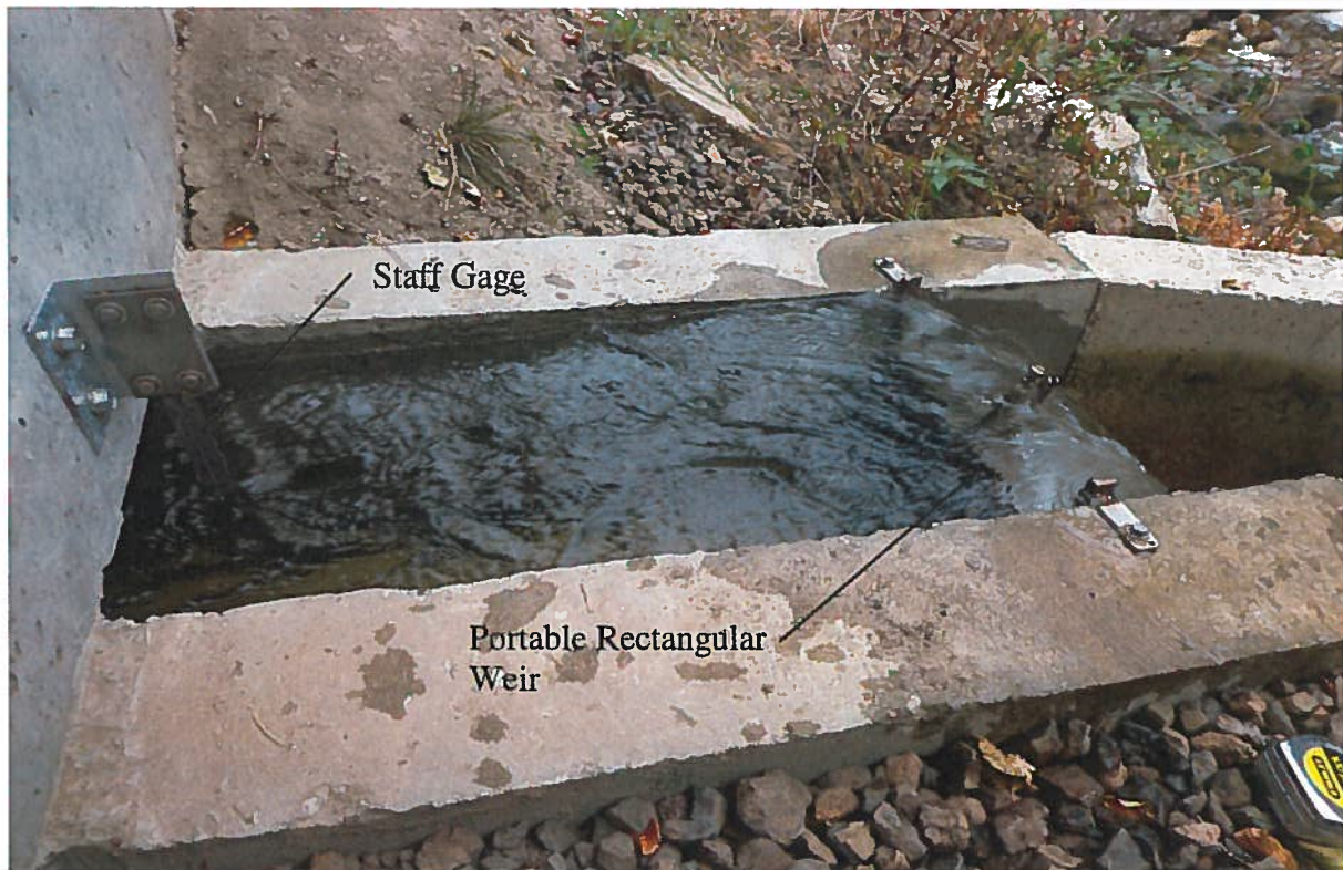
View of the 17" wide by 24" deep concrete raceway which discharges to French Creek. A portable rectangular weir is shown for flow measurement. Attached to the bracket mounted to the wall of the power station is a staff gage for flow measurements.
