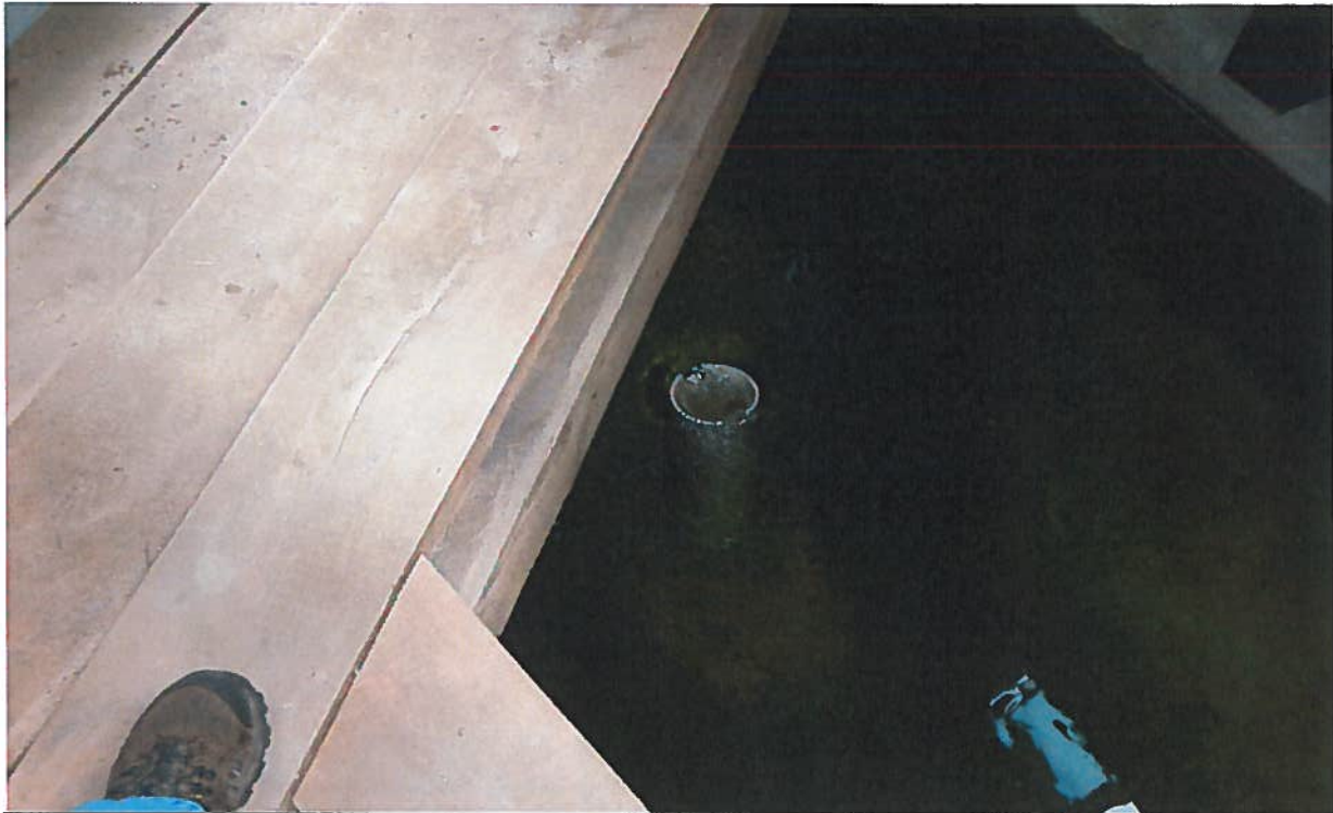
View of a section of 6" PVC vertical pipe used to control the water level in the concrete inlet channel in the penstock inlet structure. The vertical pipe is also used to divert leaves and other debris back to French Creek.
