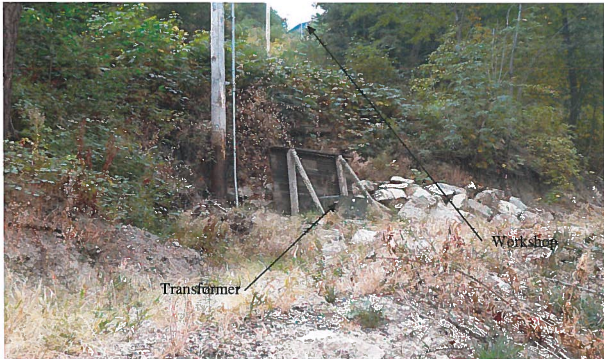
View southeasterly of the transformer for the power station. Overhead power lines deliver the electricity to the home and miscellaneous structures at the top of the hill. The corner of a large workshop is shown at the top of the photo.
