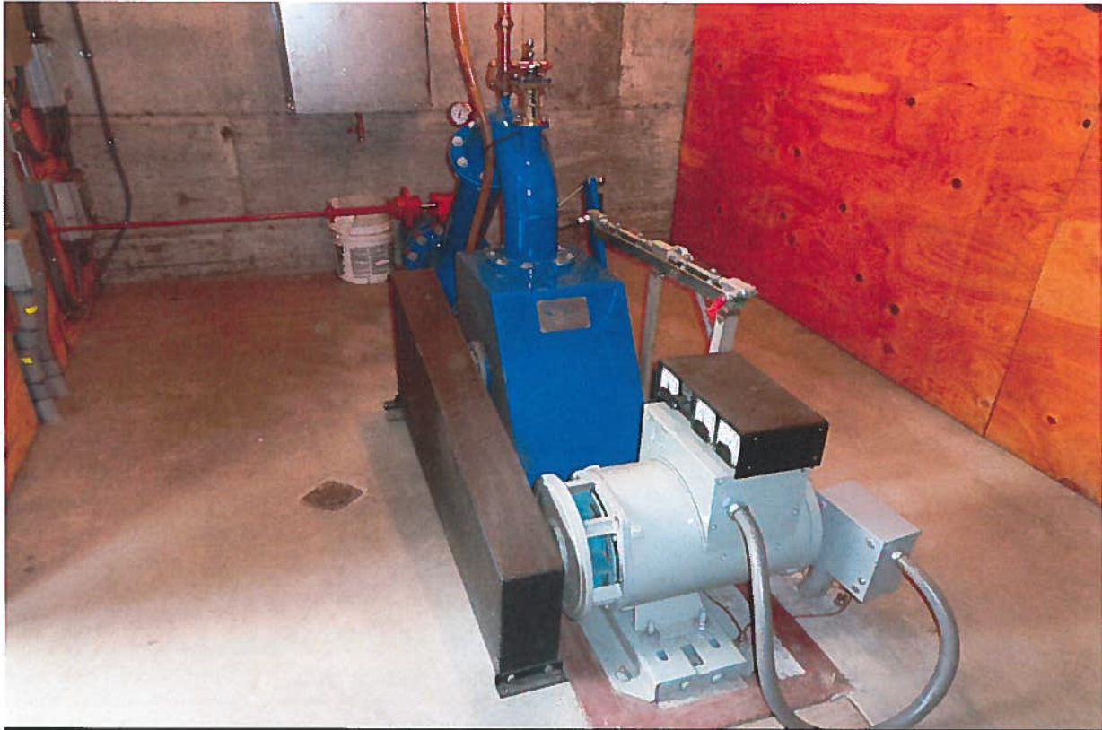
View inside of power station of the 6" penstock connection to the enclosed pelton wheel and the power turbine.
