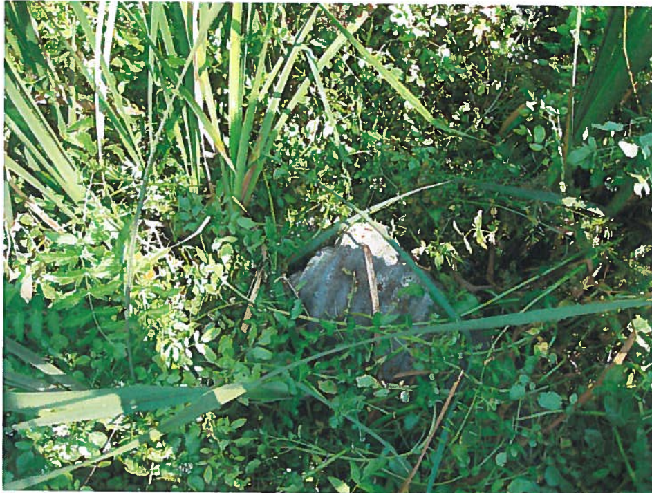
Looking at Pipe going from weir Box to COMINGLING POND
