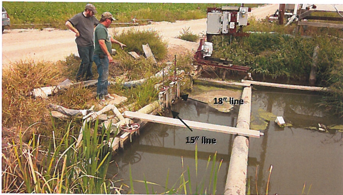
Licensed POD – Looking east at the unnamed drain showing the headgates for the 18" and 15" lines that run from the drain to the bubbler.
