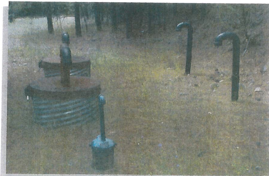
Domestic well and pressure tank vaults (vertical corrugated metal pipes) associated with — Bear Paw Campground, looking west
