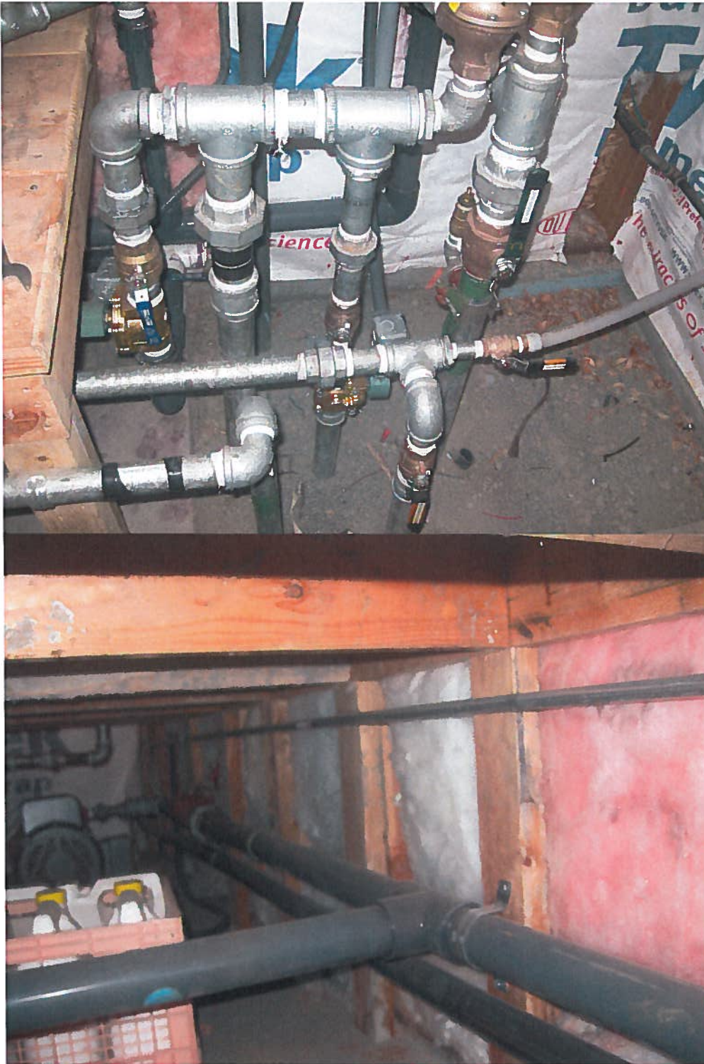
irrigation line and booster pump
