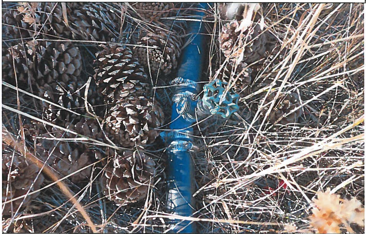
View of the 1 1/4" PVC irrigation main line and a typical irrigation gate valve for hose attachment.
