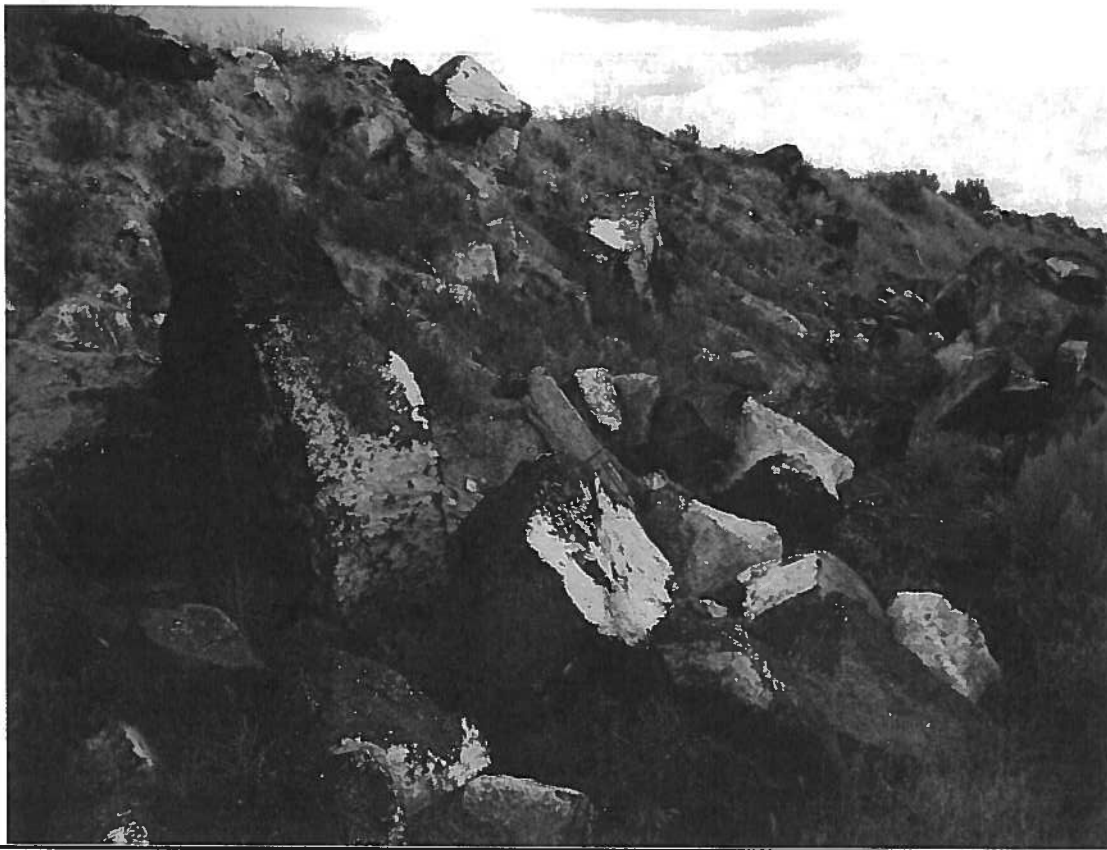
Photo of left section of embankment, riprap is gradually migrating down slope from dam crest.
