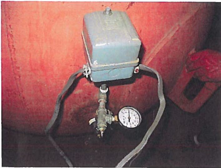
3. Pressure switch and gauge reading about 40 psi.
