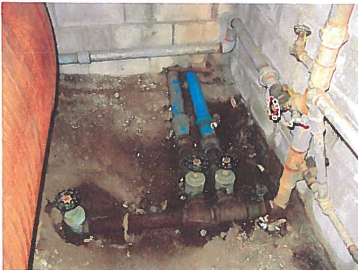
5. Distribution lines, isolation and shutoff valves.
