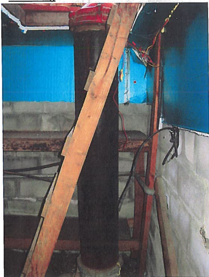
1. Well casing, well cap, and exposed wiring.
