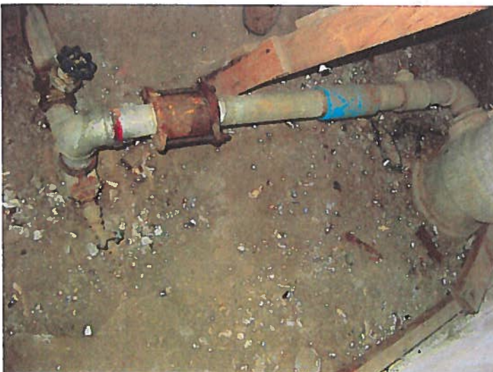
7. Accessible check valve prior to the main shutoff valve.
