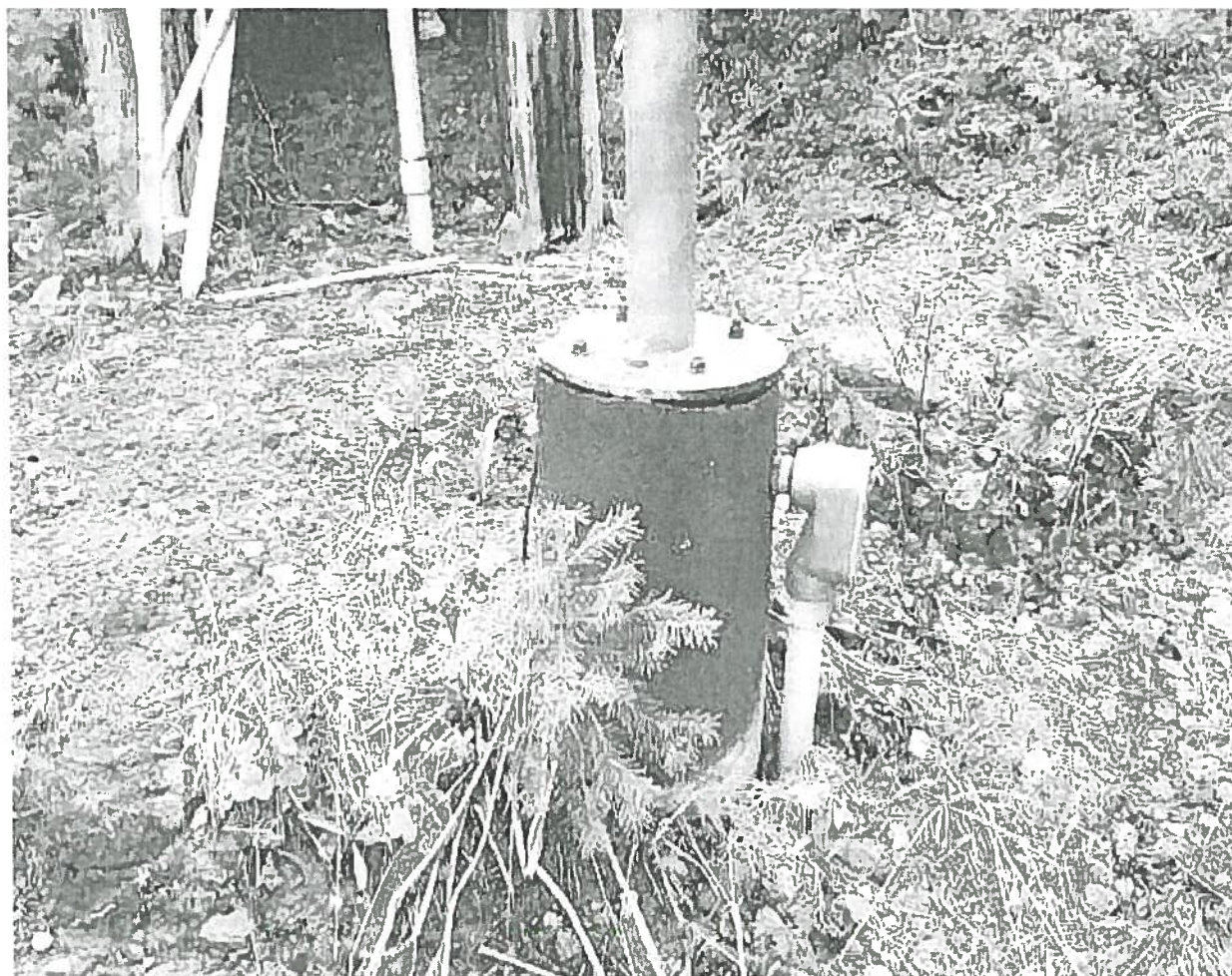
Picture No. 3; Wellhead with tag with open seal (crack).
