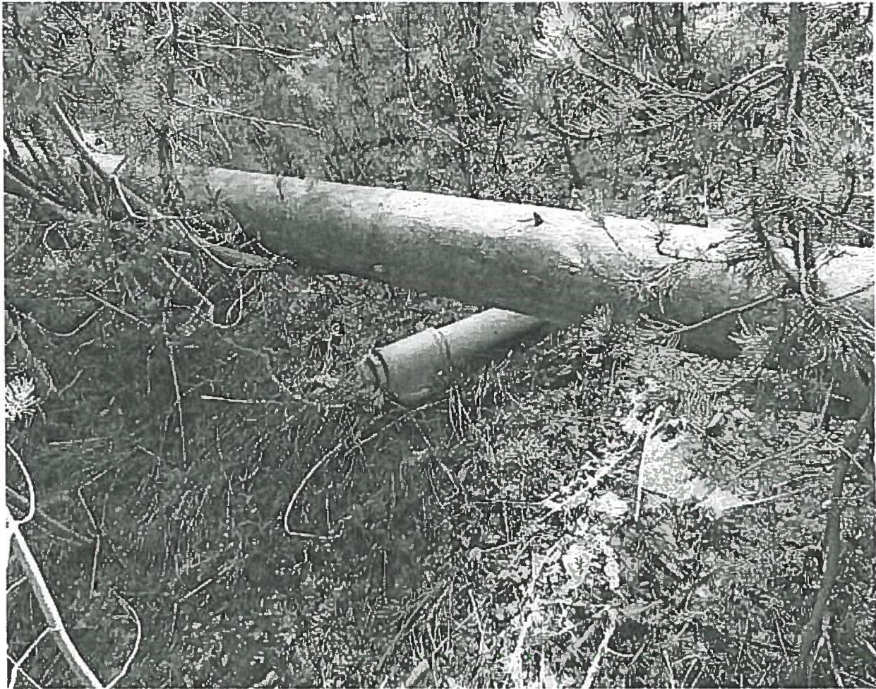
Picture No. 6; Pump to waste plug.
