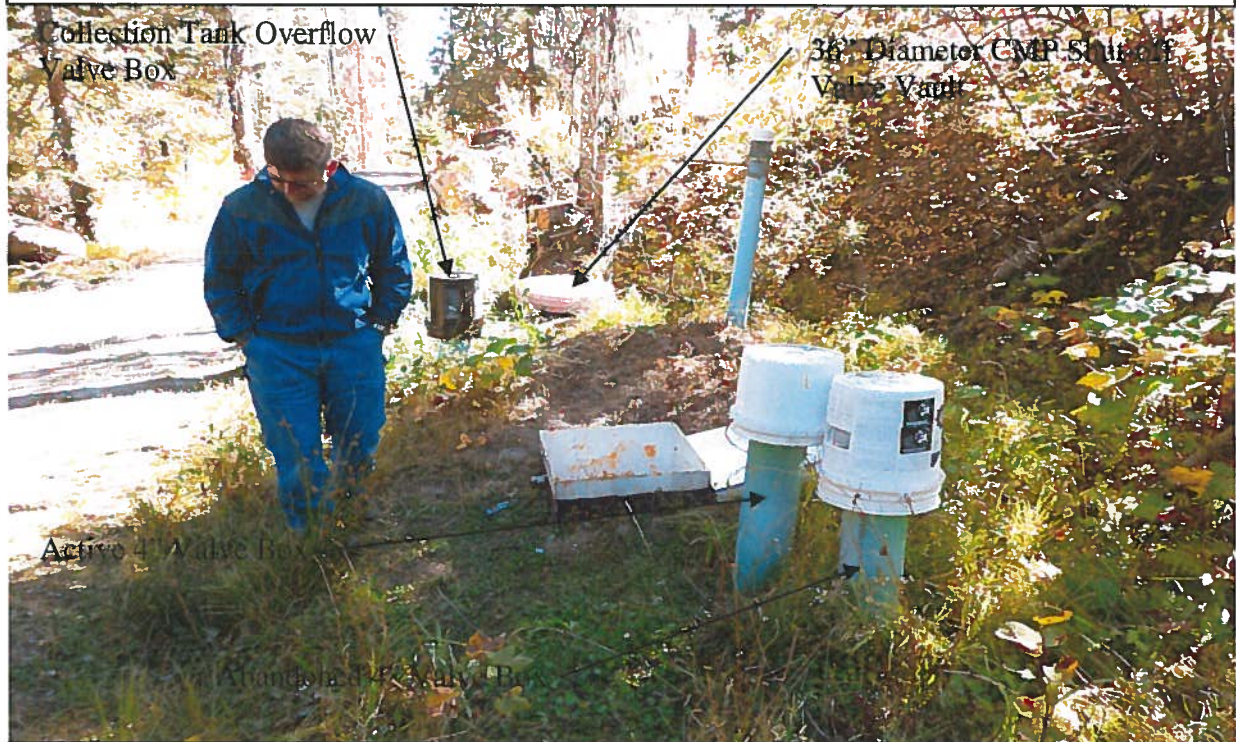
View easterly of the lid to a buried 1,500 gallon collection tank. Two PVC valve risers are shown westerly of the collection tank. The westerly most valve served the old collection system and has been abandoned. The new valve is used to regulate the flow from the settling/filter pond to the collection tank. Easterly of the collection tank is a 36" diameter CMP vault which contains the shutoff valve for the 4" PVC line to the Water Treatment Plant.
