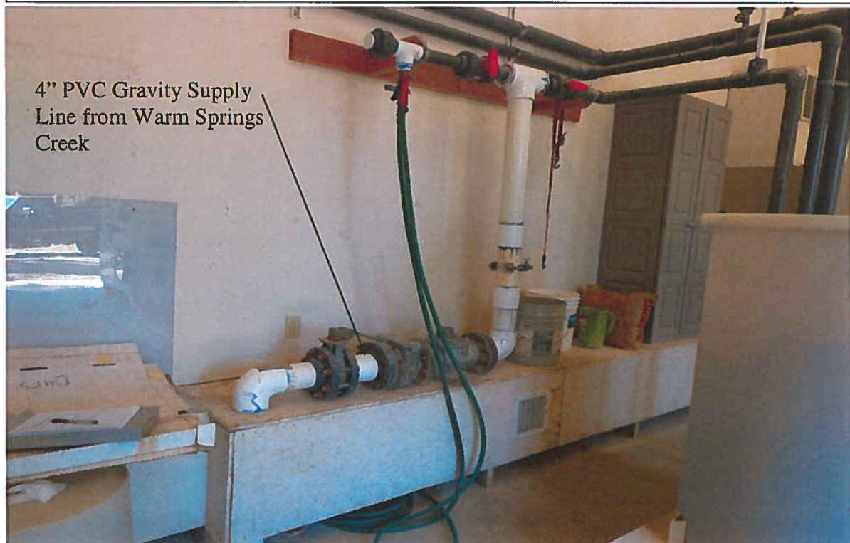
View inside of Water Treatment Plant of the 4" supply line from the Warm Springs Creek diversion facility.
