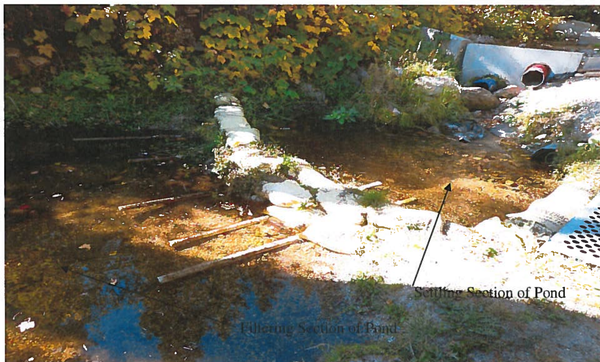
View southwesterly of the 2" PVC discharge pipes from the settling section of the pond discharging to the filtering section of the pond. The three (3) 12" CMP diversion pipes from Warm Springs Creek are shown to the right. The diversion of water through the lower 12" CMP is not controlled by a slide gate as are the upper two 12" CMP diversion pipes.
