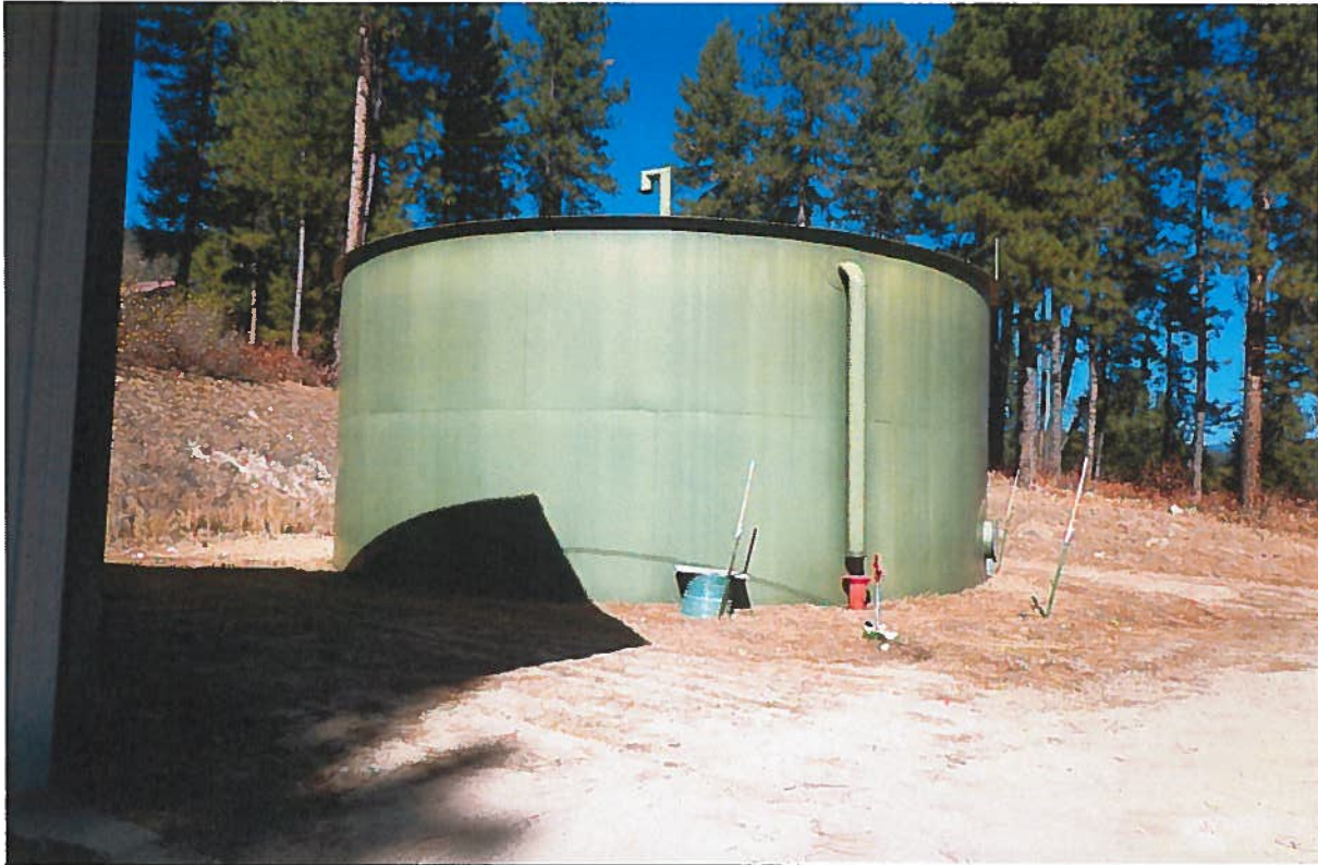
View northwesterly of the 100,000 gallon water storage tank located near the Water Treatment Plant.
