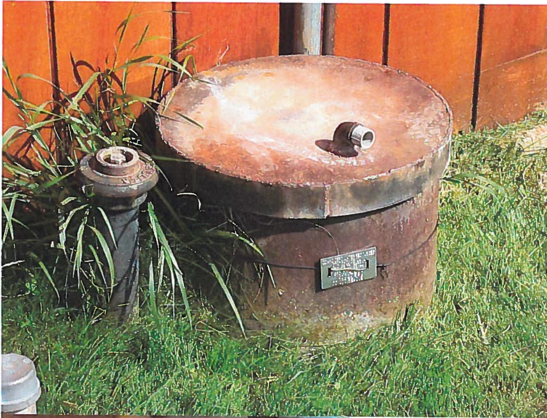
Well casing on the west side of the pump house, facing the pond
