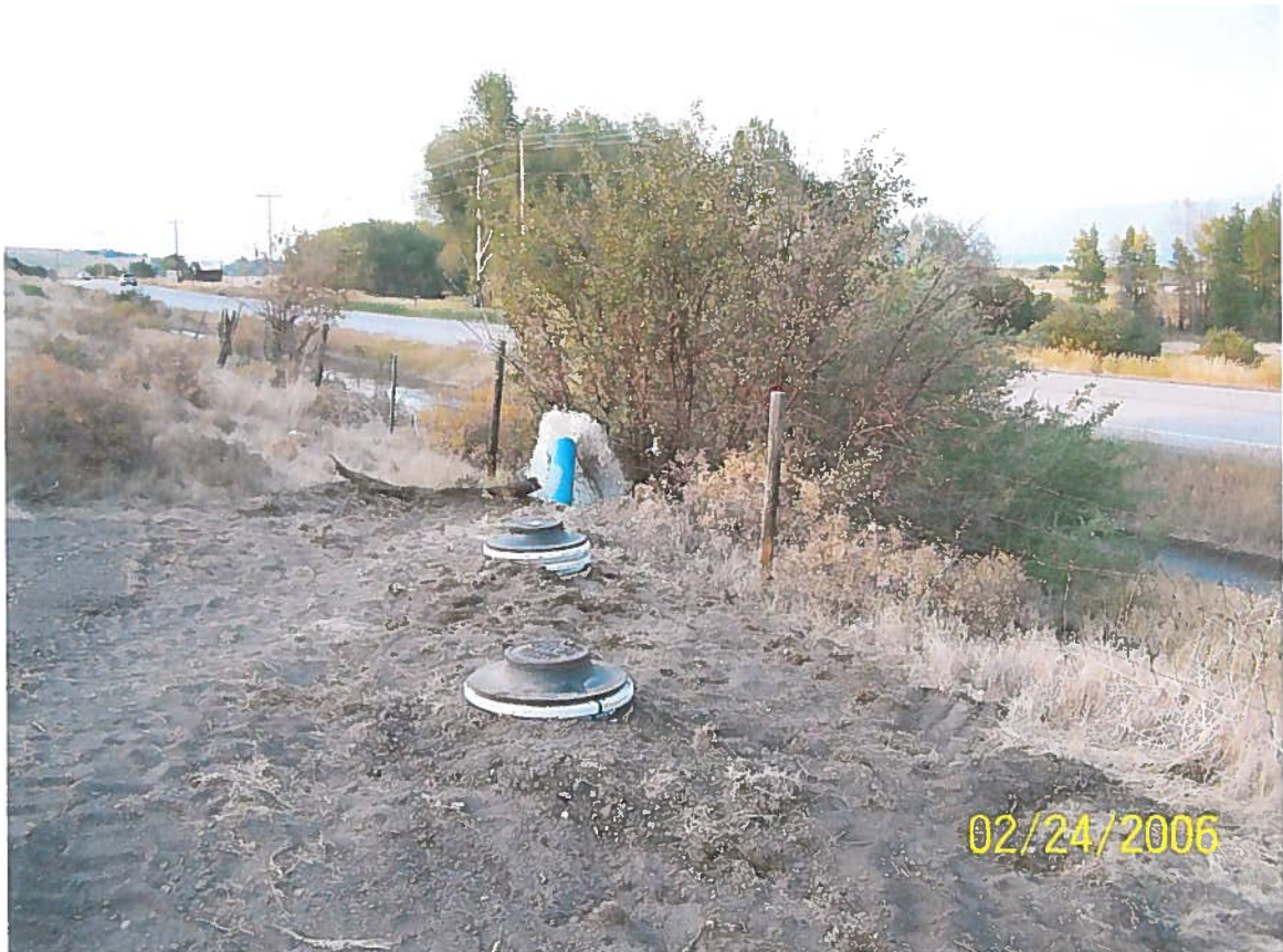
Terminus of the Sam's Hollow mitigation pipeline.
