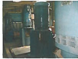
4 PUMPS AT POD 1.JPG
