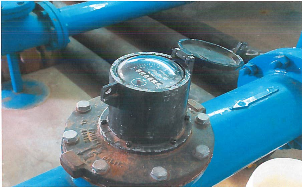
Flowmeter inside wellhouse
