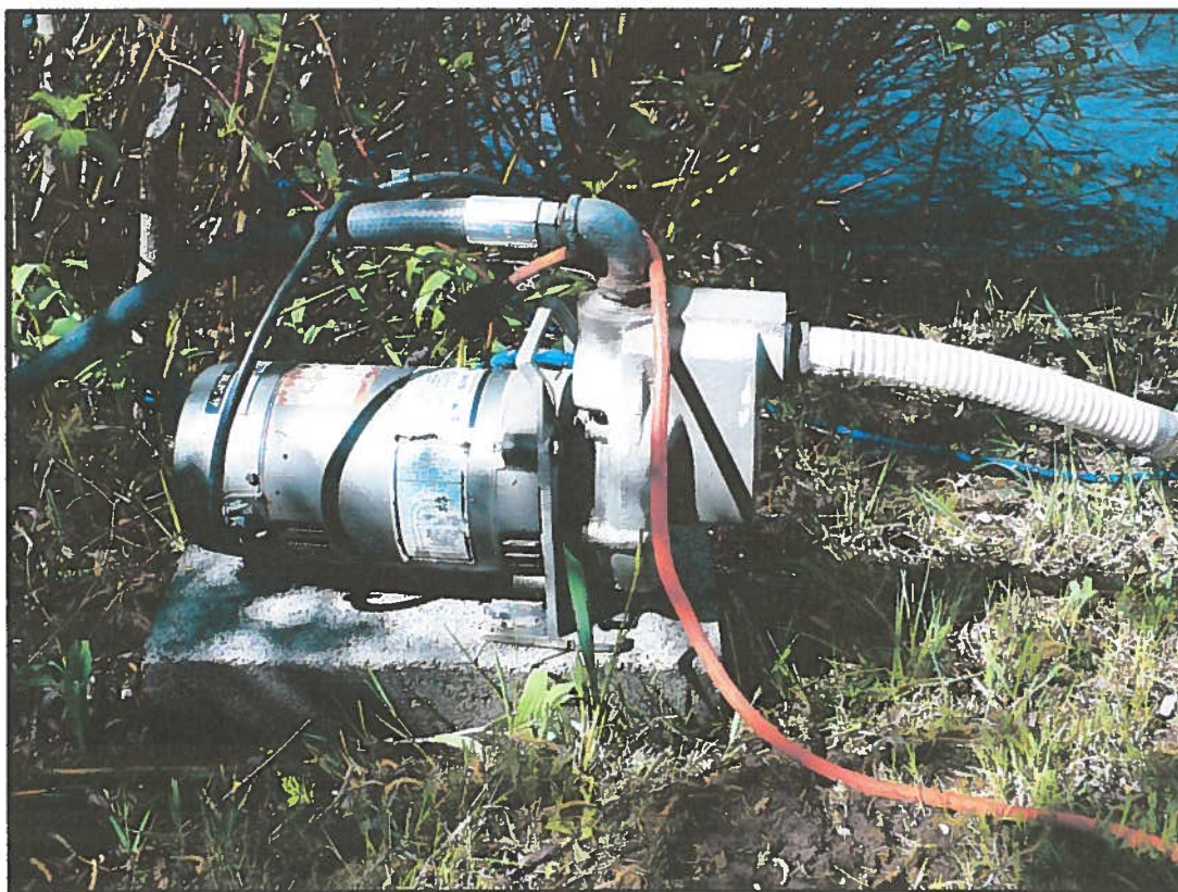
Pump at point of diversion.
