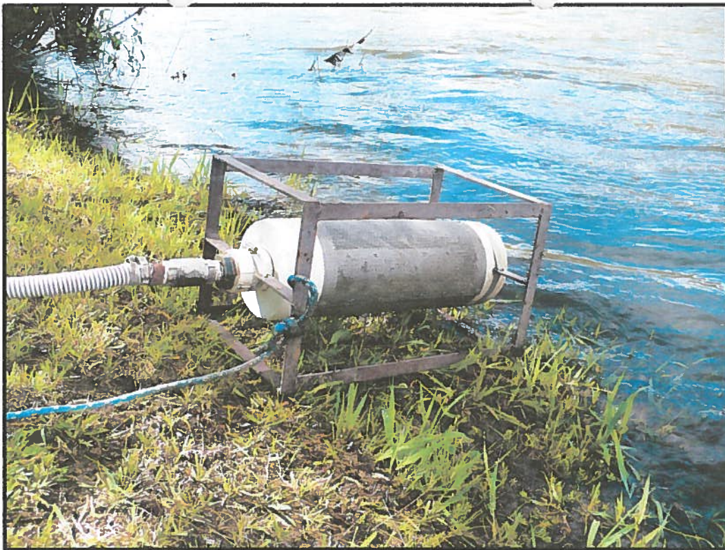
Screened foot valve.
