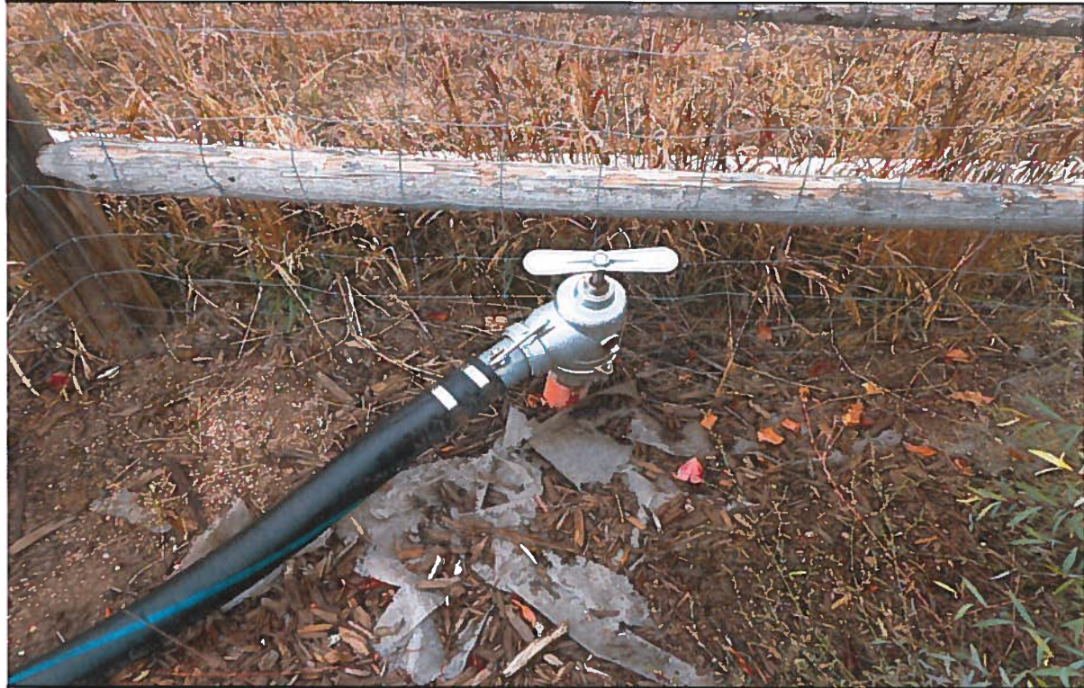
View of the 2" PVC riser and control valve at the end of the 4" PVC river supply line. The 2" PVC pipe conveys water to a sprinkler main line for irrigation of the lawn and landscaping adjacent to the right holder's home.
