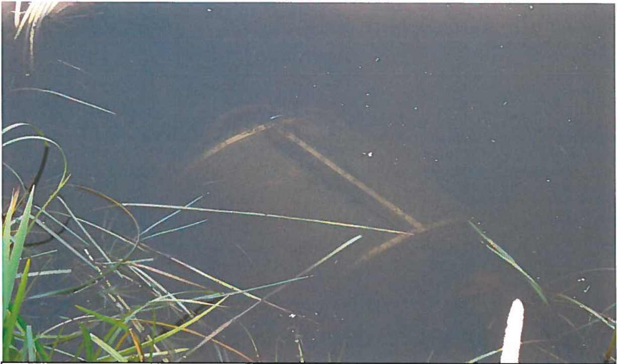
Self-Cleaning screen for 4" suction line located at the southwesterly end of storage pond. A 5 hp pump diverts water from the pond and discharges to a recirculating lined stream channel located westerly of the storage pond.
