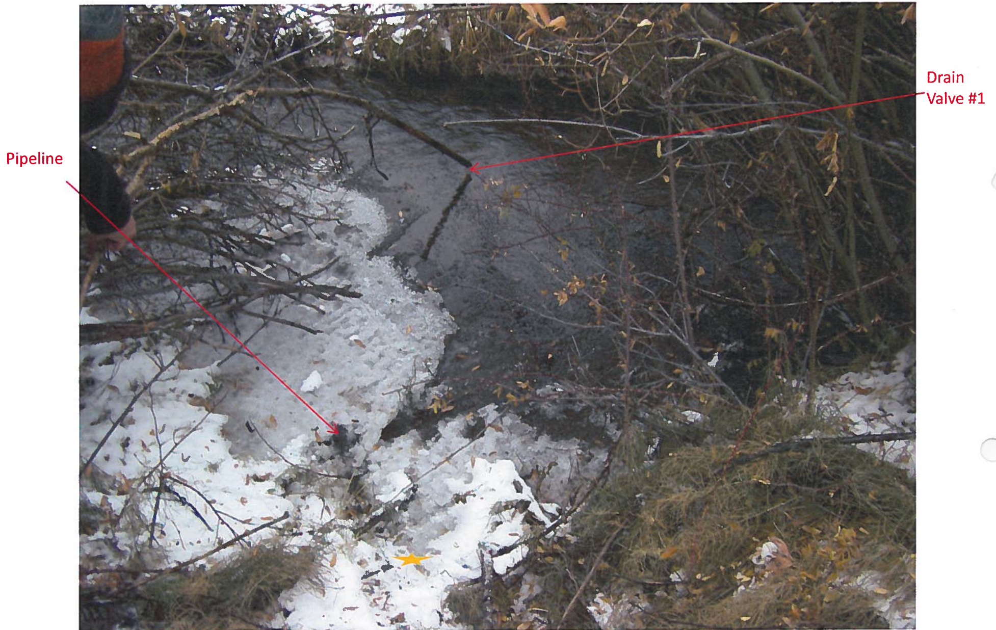
Drain Valve #1 T11N, R24E, S20, NWNW ★ N44.1881 W113.6489 (GPS)
