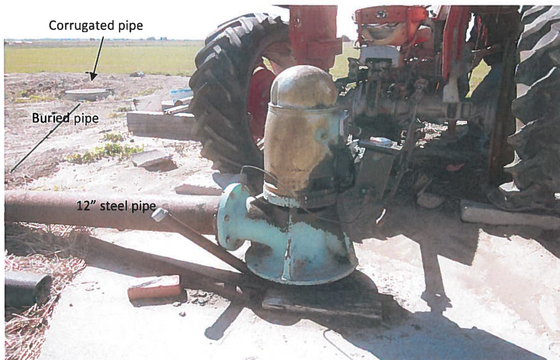
Well, PTO drive, steel pipe from well to buried 12" PVC pipe that goes to the corrugated metal pipe, see in left background.
