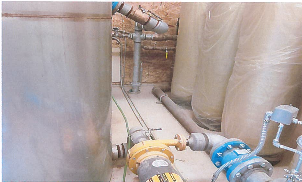
Inside the pump house.
