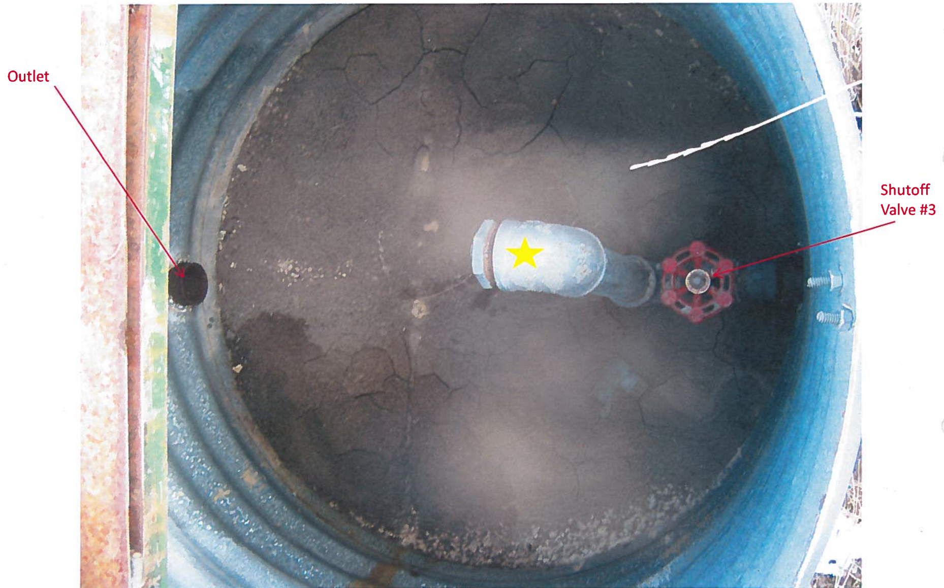
Shutoff Valve #3 T13N, R22E, S19, SWNE ★ N44.4429 W113.8993 (GPS)
