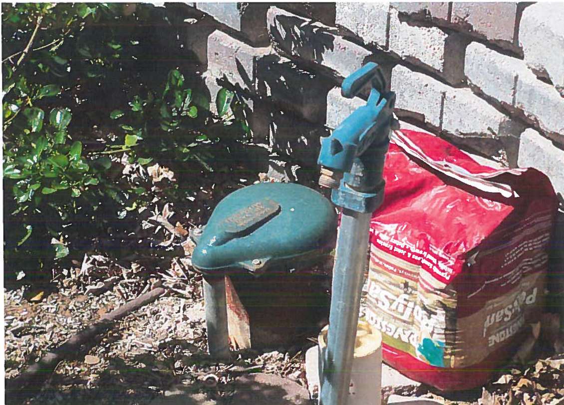
Wellhead and Outdoor Faucet
