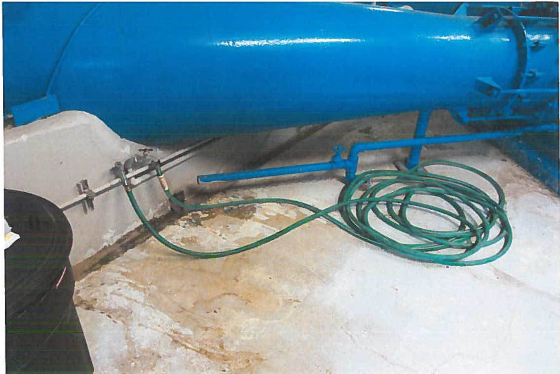
Faucet and hose used for washing interior of powerhouse
