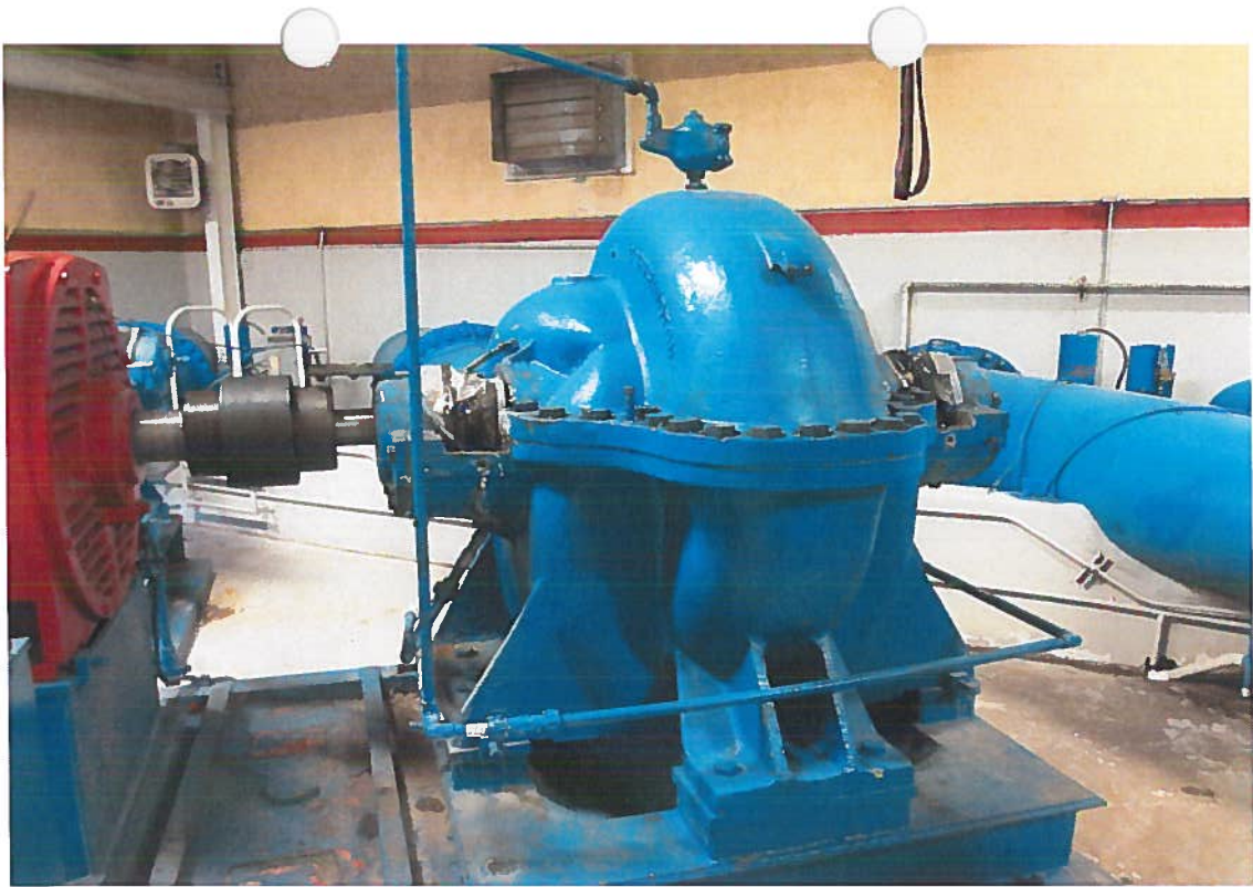
View of turbine and interior of powerhouse
