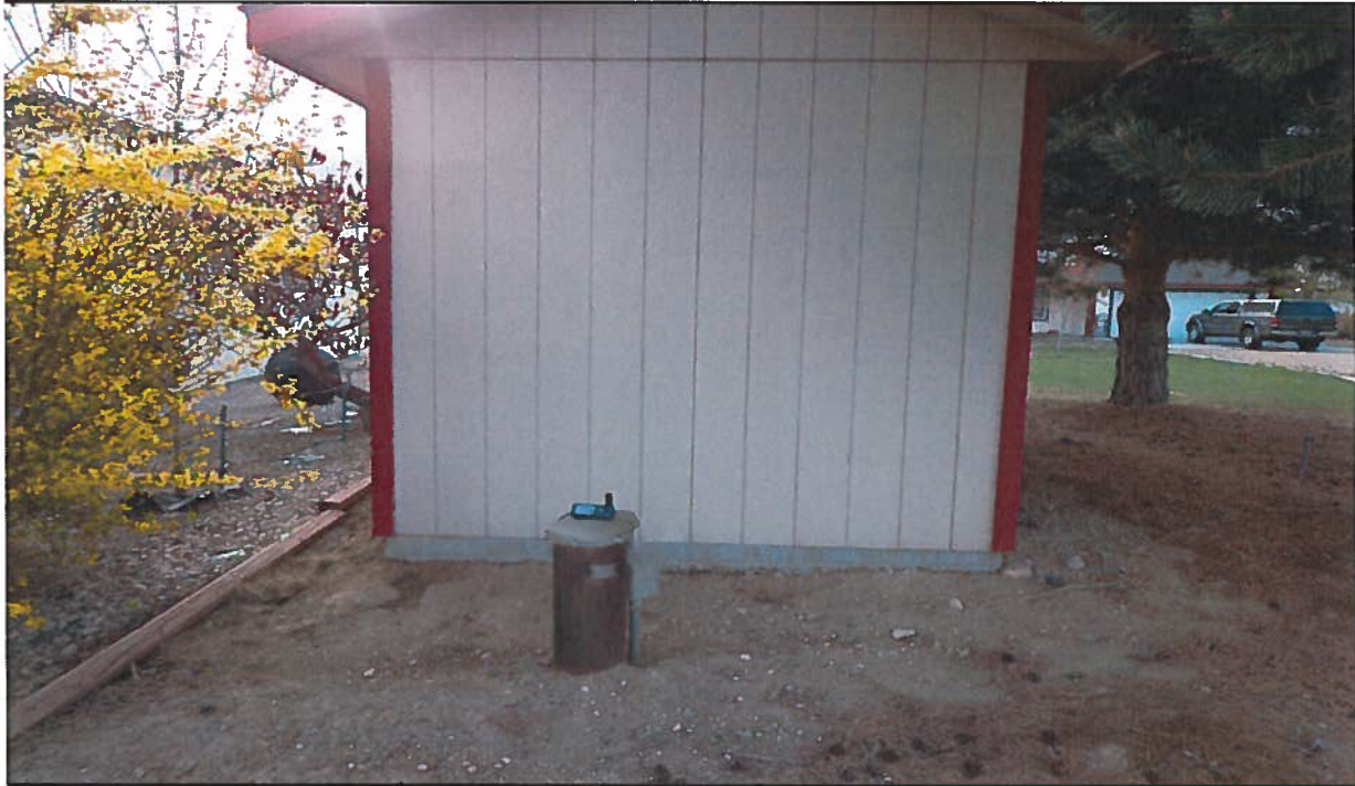
Point of Diversion: View easterly of the ground water well and pump house. The well and pump house are located within Lot 4, Phase 2, of the Willis Ranch Subdivision.
