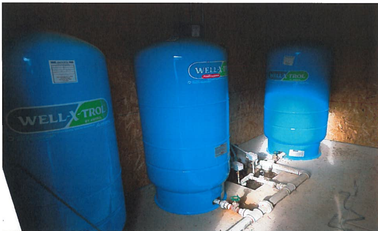
View inside pump house of the three (3) pressure tanks, pressure switches, and discharge piping. Two pressure switches exist due to the two (2) 2-hp submersible pumps in the 8" well.
