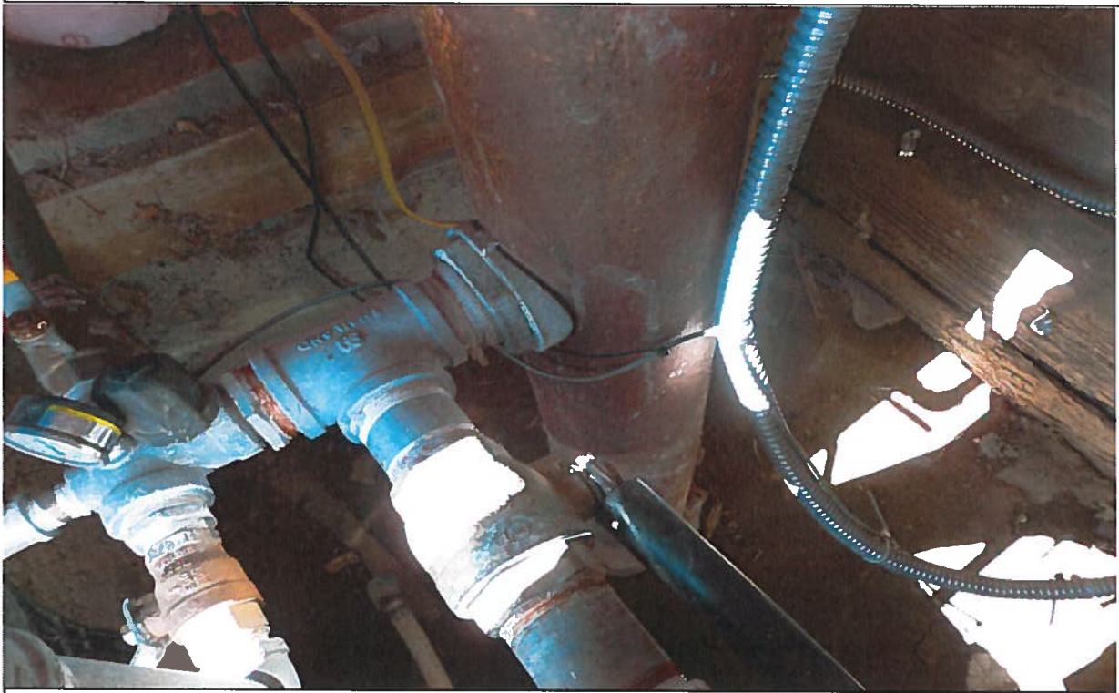
Point of Diversion: View inside pump house of well and discharge piping.
